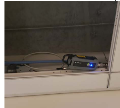
Use of iVA in a DAS job.
